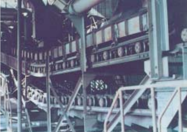
Long pan conveyor
