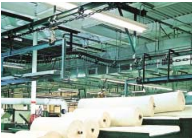
Trolley conveyor system
